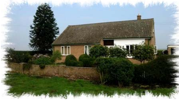
10m high monkey puzzle tree situated about 5mtrs from the damaged bungalow.
